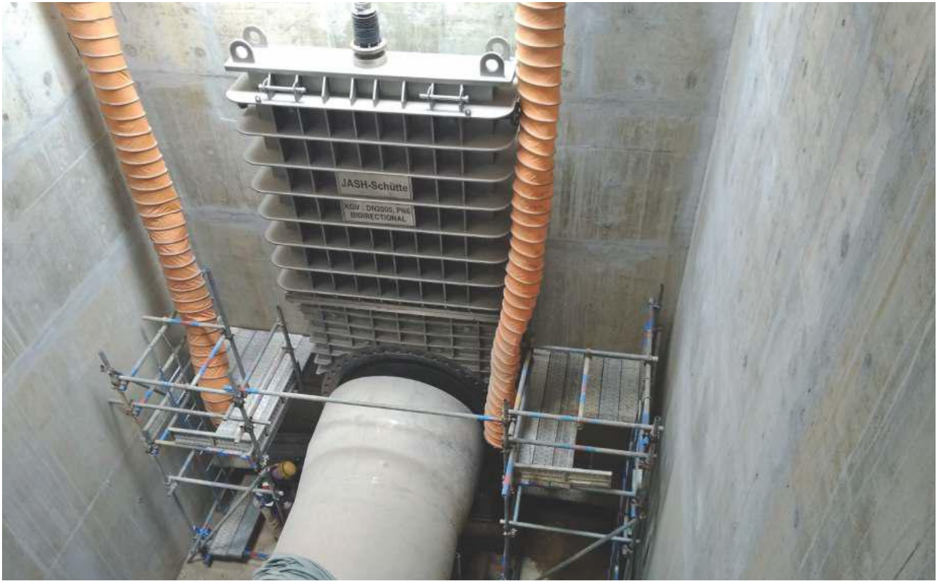
Installation of Bidirectional DN 2000 (80"), supplied to PUB Singapore for Changi Water Reclamation Plant
