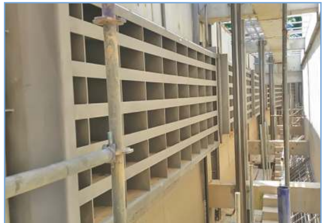
5000 x 1900 mm Stainless Steel Weir Gates at Stamford Canal, Singapore
