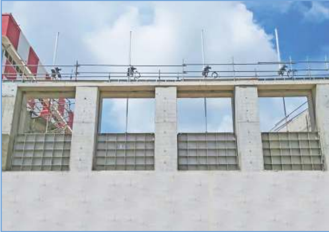
3000 x 2400 mm Stainless Steel Sluice Gates at Changi Retention Pond, Singapore
