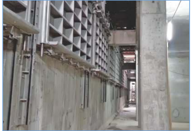
3000 x 2000 mm Stainless Steel Weir Gates at Happy Valley, Hong Kong
