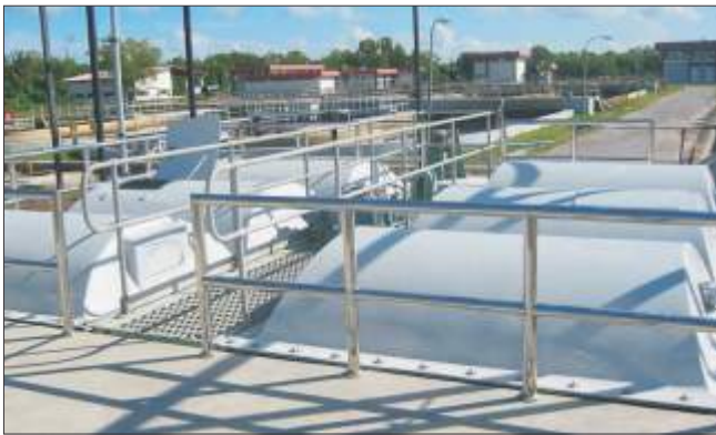
Detritor Mechanism with FRP Hood- STP at Brunei
