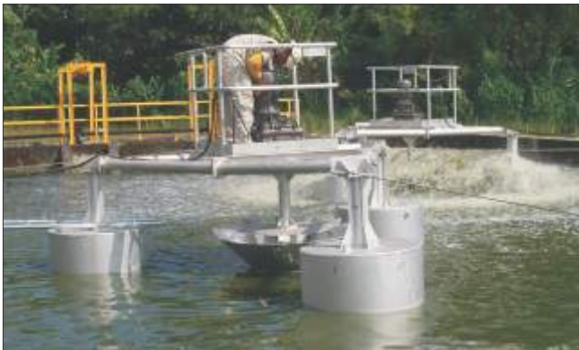
Slow Speed Floating Aerators at Ipoh STP, Malaysia
