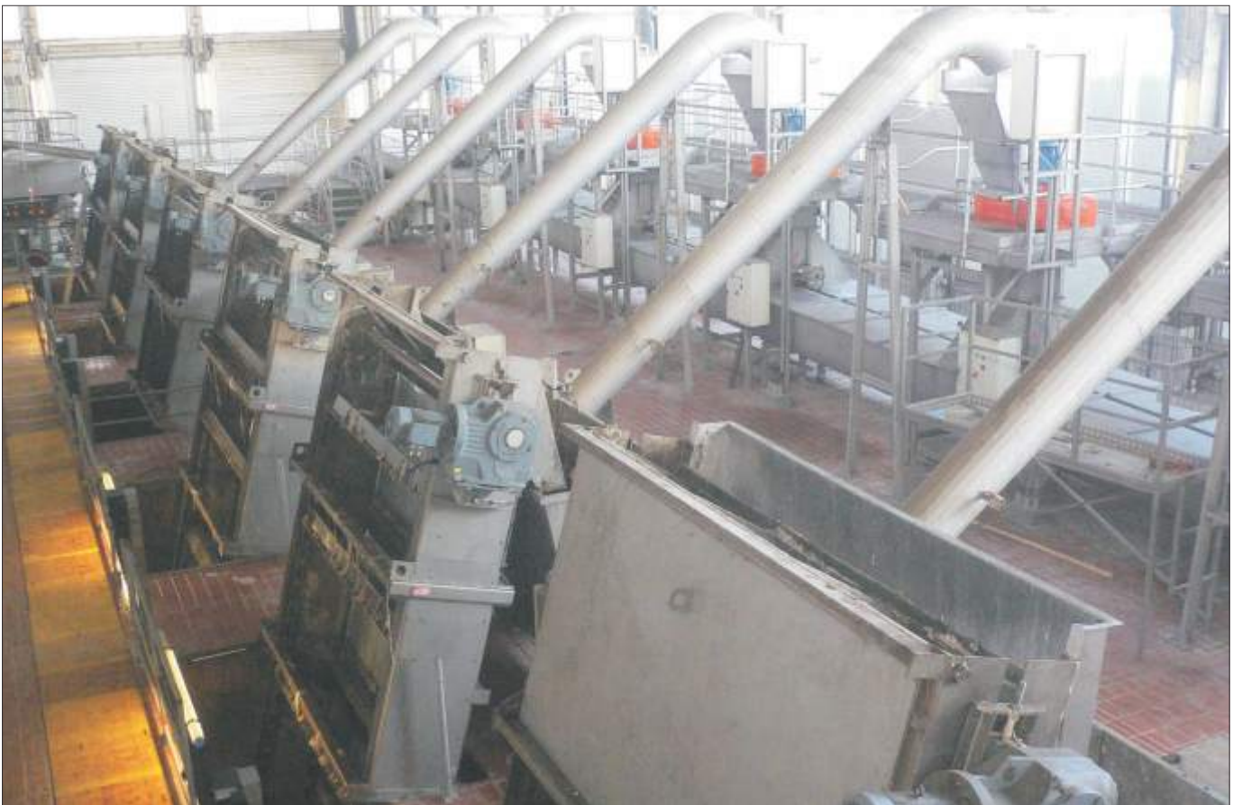
6 Nos. Multirake Screens with 3 to 6 mm (0.12” to 0.24”) spacing at Vienna Main Sewage Treatment Plant
