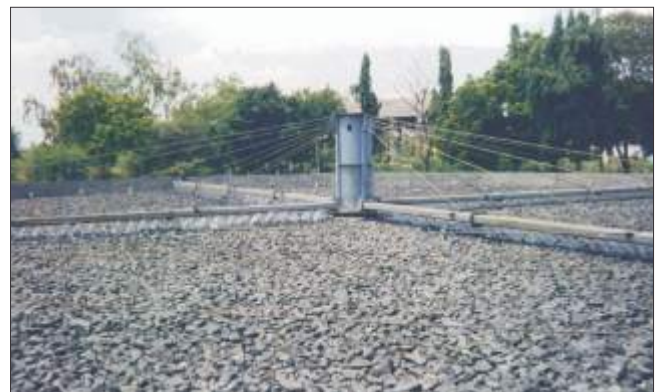
48m (158') Diameter Trickling Filter at Baroda STP, India
