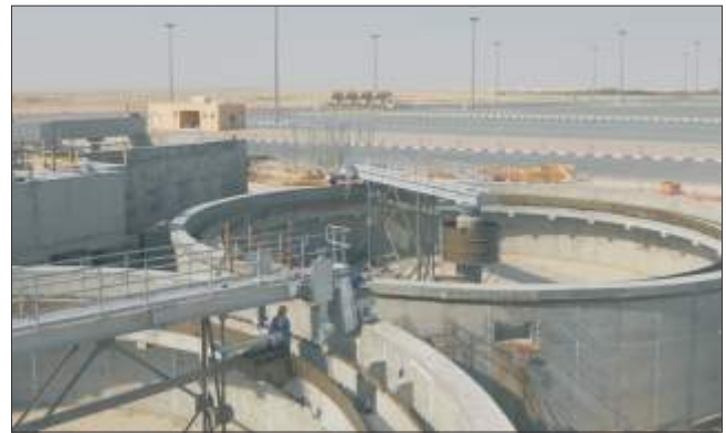
Peripheral Driven Traction Clarifier at Doha STP, Qatar
