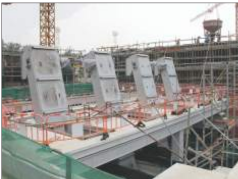
MM2MM™ Multirake Screens at Pillar Point STP, Hongkong
