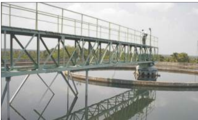
45m (148') Diameter Clarifloculator at Cochin Refinery, India
