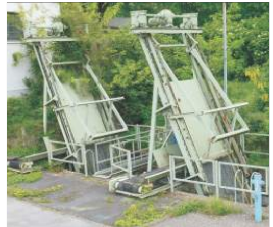
Screen installed in 1927 and still operative
