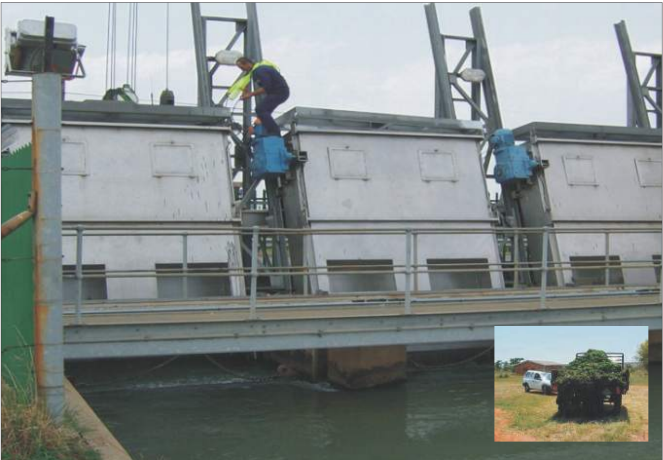
“MM2MM”™ Multirake Screen Installed at Zuikerbosch WTP
