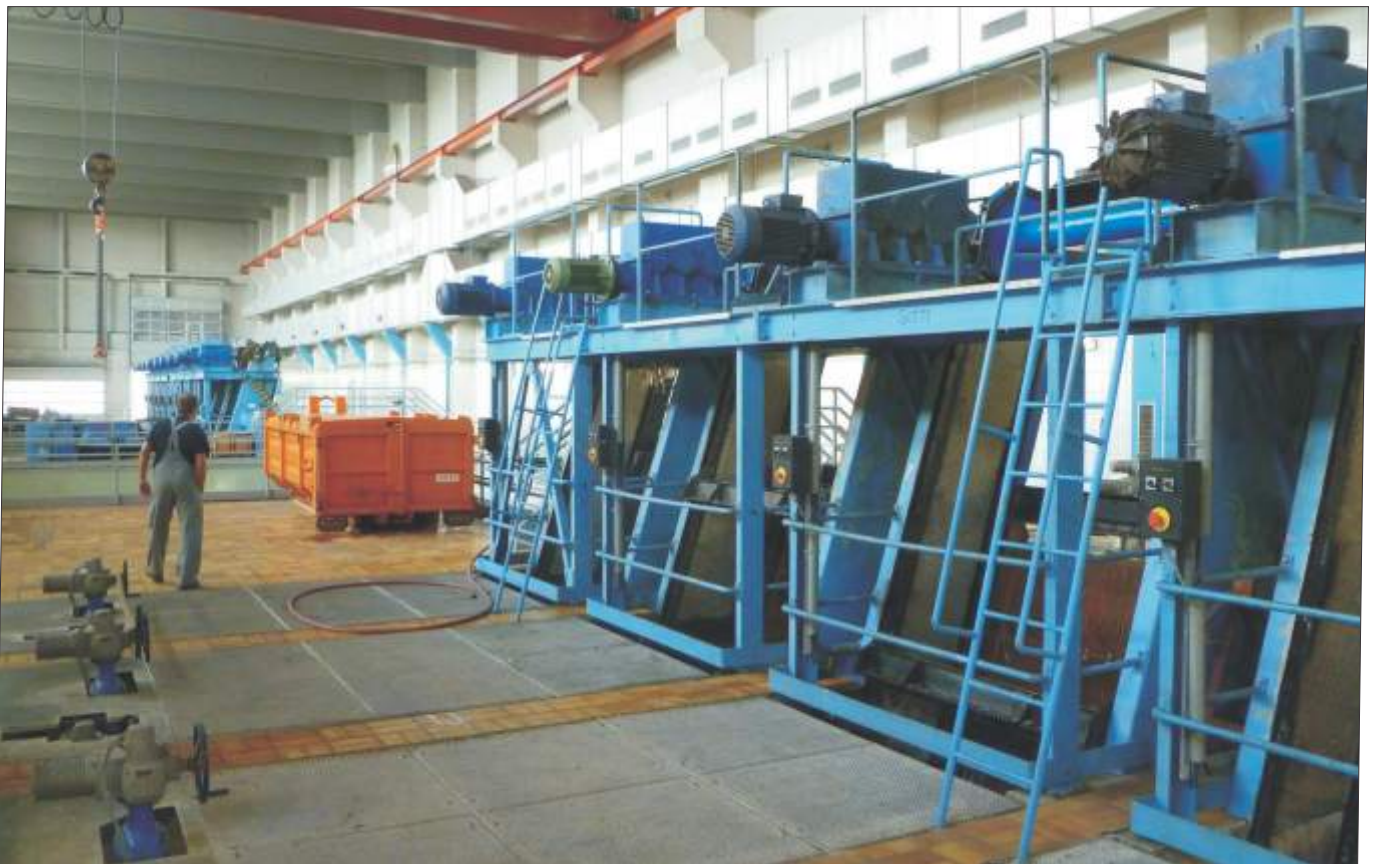
Screens Installed in 1978 at Vienna Pumping Station
