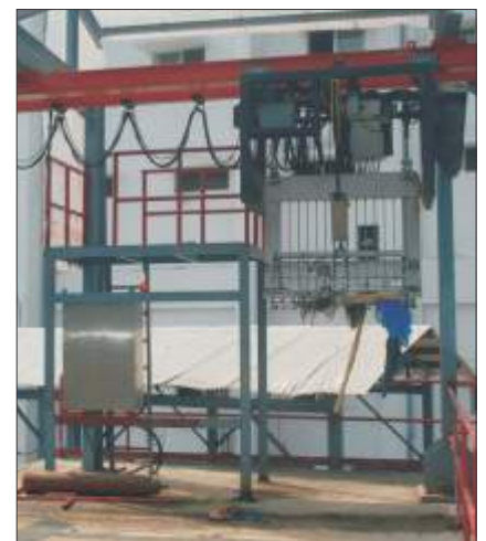
Carriage Maintenance Station with Control Panel
