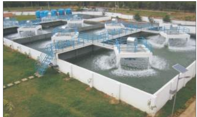
Slow Speed Fixed Aerators at Bangalore STP, India
