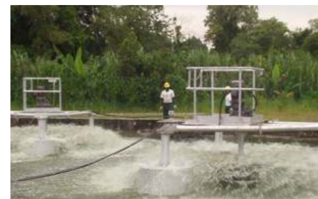
Slow Speed Floating Surface Aerator Type SP-SA-2 IPOH STP, Malaysia
