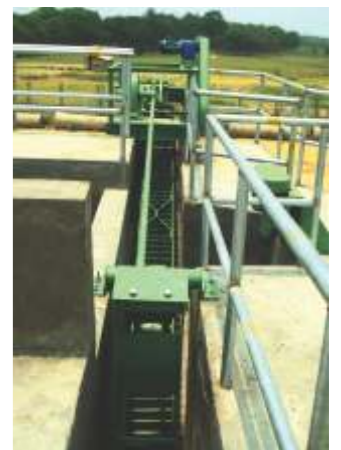
Rake type Classifier Assembly 50MLD STP, Chandigarh
