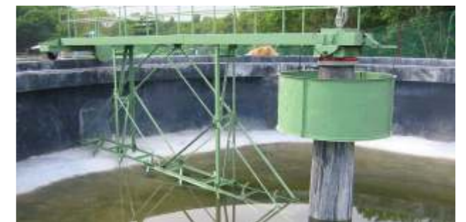
Type SPC-B 21m dia Peripheral driven Traction Clarifier at Crimson STP, Malaysia.
