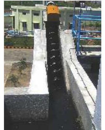
Screw Classifier Assembly Nagole STP, Andhra Pradesh
