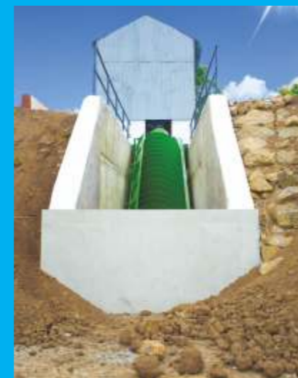
18.5kW Hydropower station at IMC, Indore
