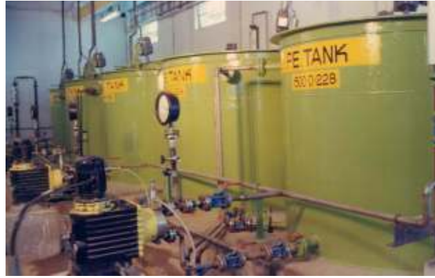
Chemical dosing station – PT Poly prima –Ciligon, Indonesia.
