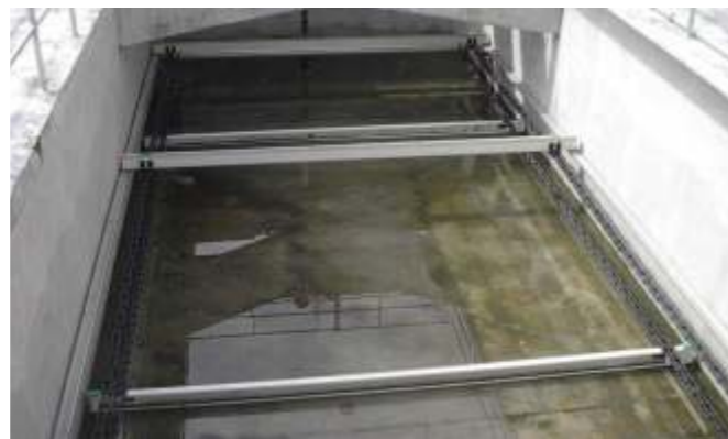
Type SP-STD: Rectangular Clarifier, Kuantan STP, Malaysia
