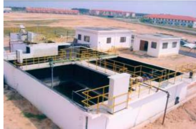
STP at Parit Bunter – West Malaysia
