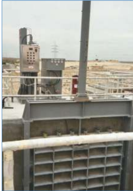
2750 x 2750 mm Cast Iron Slide Gate with Hydraulic Actuation Waste Water Pumping Station, Alexandria, Egypt
