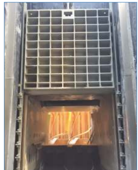
2500 x 2500 mm Cast Iron Slide Gate at HATS2A Project, Hong Kong
