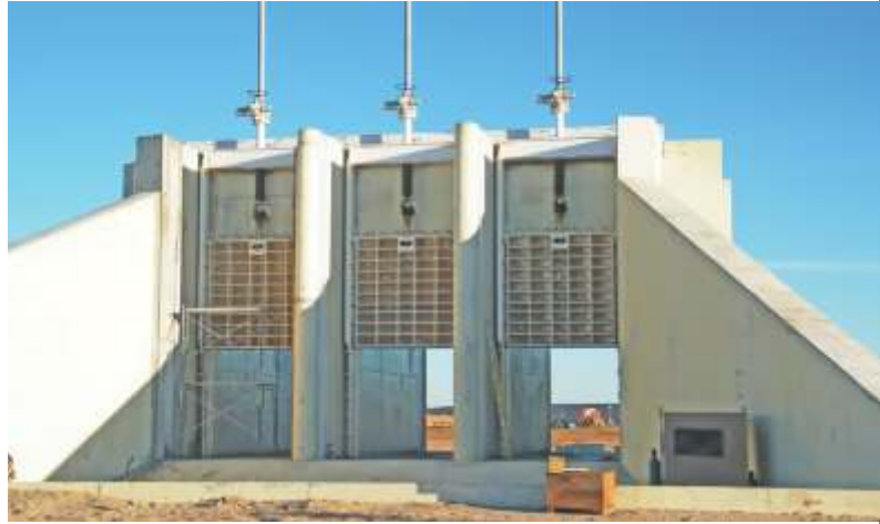
3000 x 3000 mm Cast Iron Slide Gates Drop Structure #2, Colorado River, CA, USA
