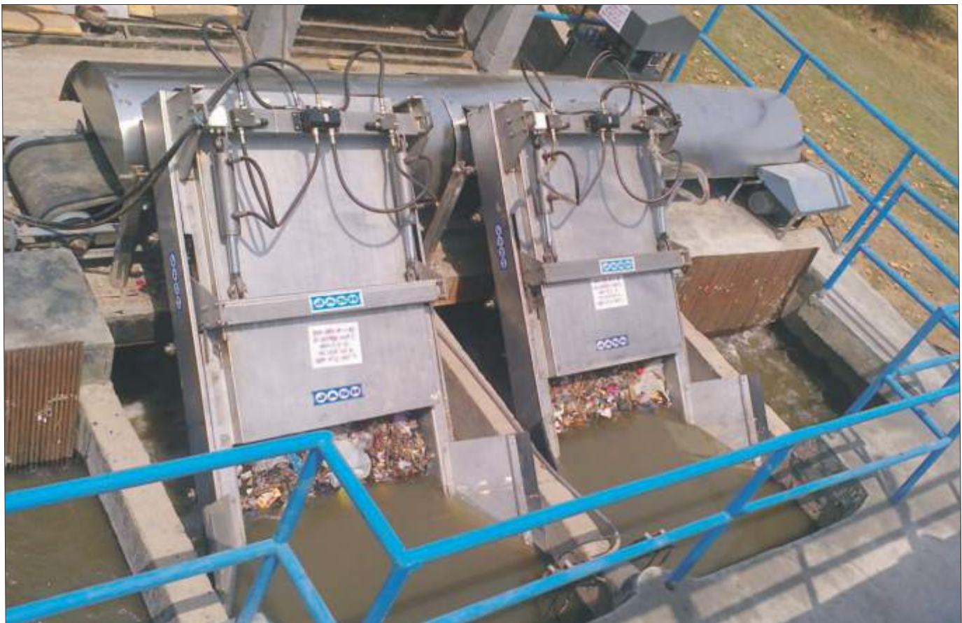
2 Nos. Screenmat Installed at 36 MLD Indrapuram STP, Gaziabad, India
