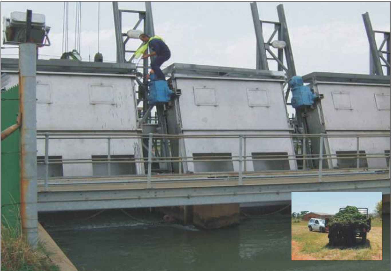
“MM2MM”™ Multirake Screen Installed at Zuikerbosch WTP
