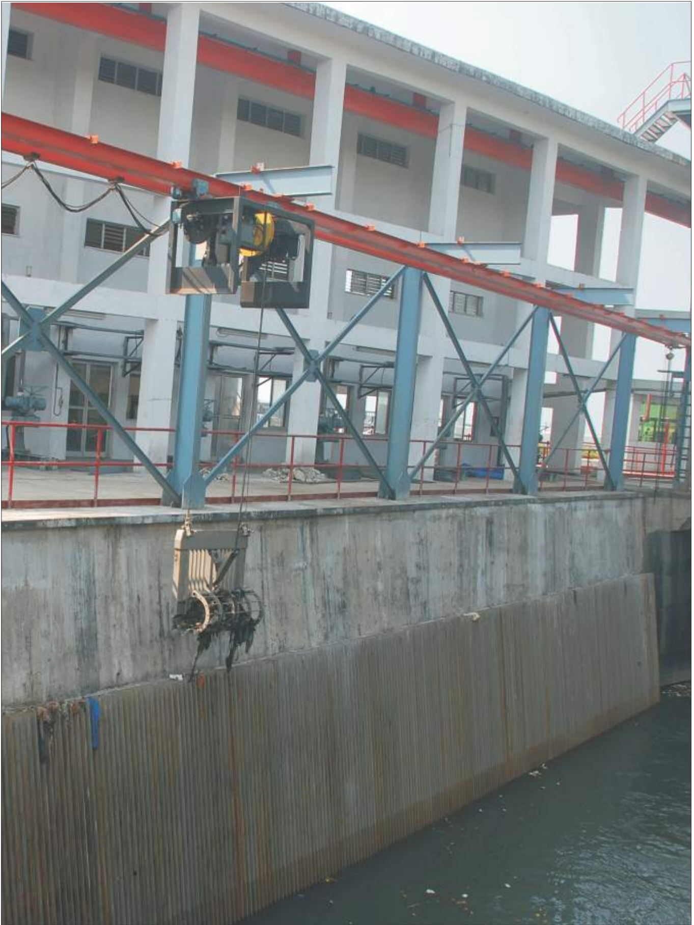
40 m (132') wide Suspended Grab Screen at 60 Cumecs Capacity Haji Ali Storm Water Project, Mumbai, India
